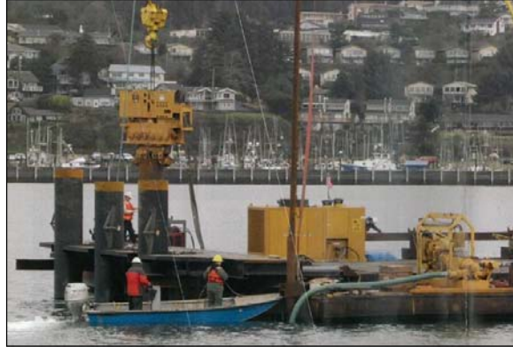
Pile driving template at the front of the barge. The template was hydraulically positioned using GPS and piles were then installed three at a time.
