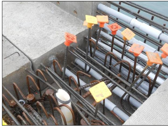
Cast-in electrical conduits at the bull rails. Conduits are coupled prior to installation of field rebar in the bent cap and topping slab.1
