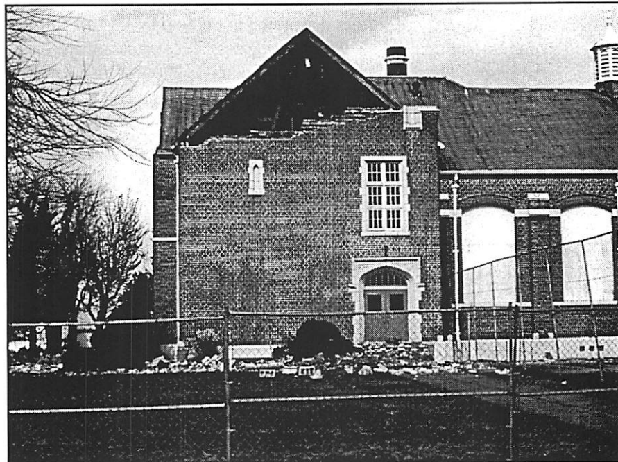
Figure 5. Photo of damage to Molalla High School, Oregon, from the Scotts Mills earthquake of 1993. Bricks from the URM gable over the doorway fell on the steps and sidewalk during the earthquake.
