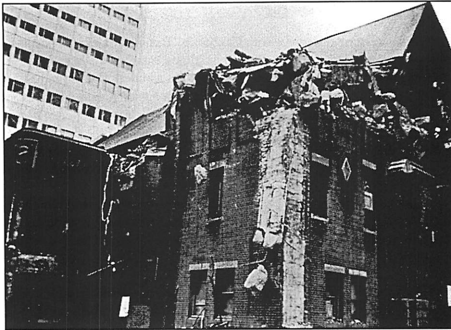
Figure 4. Damage to a URM church in the January 17, 1995, earthquake in Kobe, Japan. Photo courtesy Japan Society of Civil Engineers, from their collection entitled "Records of the 1995 Great Hanshin-Awaji Earthquake Disaster."
